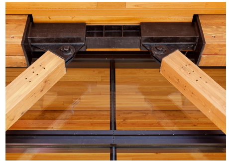
Special care was taken in connection design, for fasteners that were both artful and able to withstand seismic activity.
